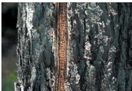
Figure 3.65. Seams are fully compartmentalized. If internal decay is present, check shell thickness.
