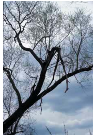
Figure 5.4. Remove large branches that are broken or lodged in the crown.
