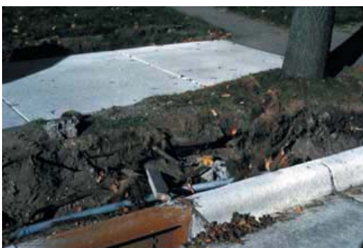
Figure 5.27. This tree has experienced damage to two sides of the root system and surface root loss due to re-construction activities. An older sidewalk restricts the roots on a third side of the root system, making this tree a prime candidate for failure.
