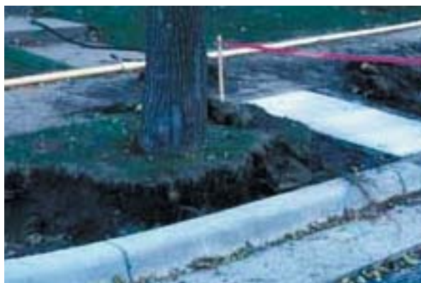
Figure 4.2. Tree with excessive root severing caused by curb and sidewalk reconstruction damage. Root severing can compromise the structure of a sound, healthy tree and increase its susceptibility to windthrow during wind loading events.
