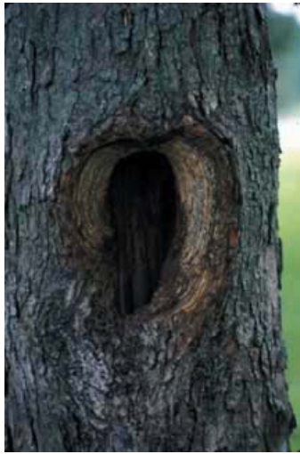
Figure 3.12. Hole in stem revealing internal column of advanced decay.
