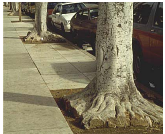
Trees roots have been cut to avoid sidewalk damage. This is a recordable damage.
