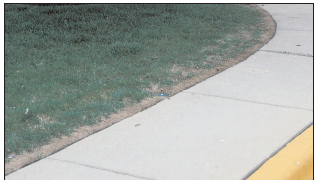
Turf along the sidewalk edge has been killed back by de-icing salts.
