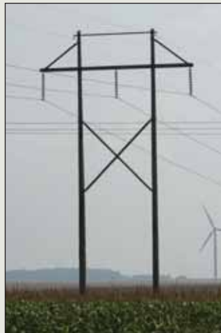
230-kV/345-kV H-frame transmission structure
