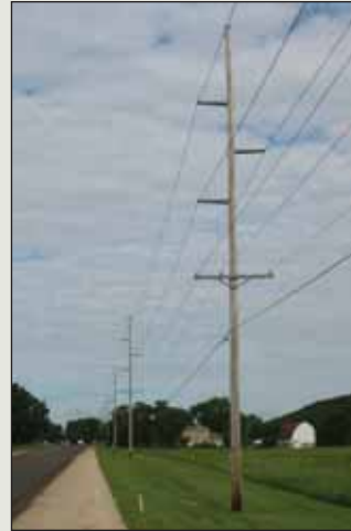
69-kV/115-kV transmission structure with distribution underbuild
