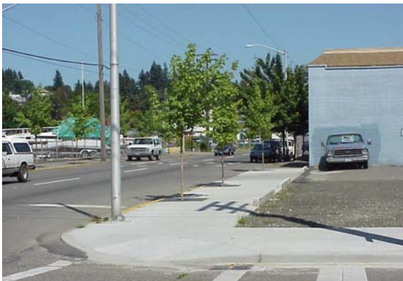
Trees installed in structural soil. South Side of State Avenue, looking East
