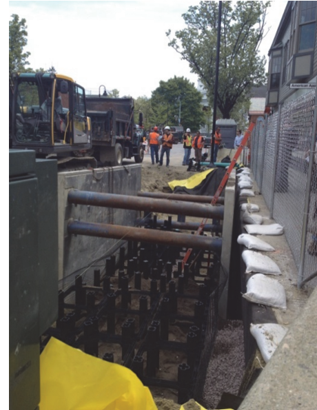
Figure 4. A structural cell system under construction on Cherry Street in Burlington, VT.
