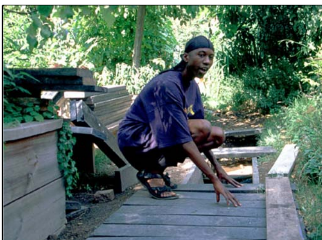
Figure 44. Gerald Brinson, who started as a volunteer for the park and is now part of the staff, describes the new dock project with flowing water that he is constructing.
