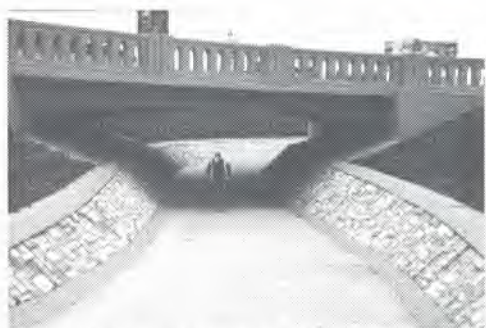
A new bicycle underpass at a freeway on-ramp in Eugene, Oregon. Attractive, safe bicycle routes play a part in encouraging greater bicycle ridership.
