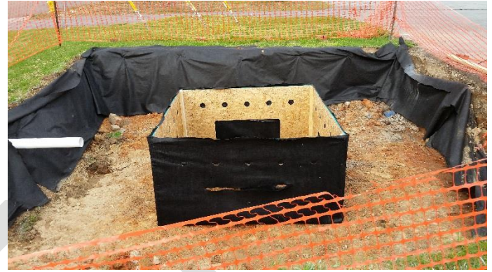
Figure 6 18'x18'x3' excavated pit next to parking lot lined with non-woven geotextile fabric. A 4" PVC drain line was installed to allow excess stormwater to drain from the system.
