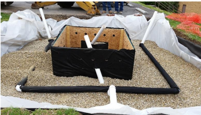
Figure 7 Under-drain constructed of 4" perforated PVC pipes, wrapped with black filter fabric, and connected to the previously installed drain line. An upturned elbow was used to regulate the amount of stored water in the system. The angled, white PVC pipes were not part of the drainage system.
