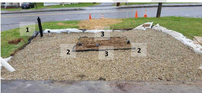
Figure 8 Location of monitoring equipment (left) and finished project (right). Perforated PVC gravel bed monitoring well (1); mini-rhizotrons in the mineral bed (2); mini-rhizotrons in the mineral/gravel interface (3).
