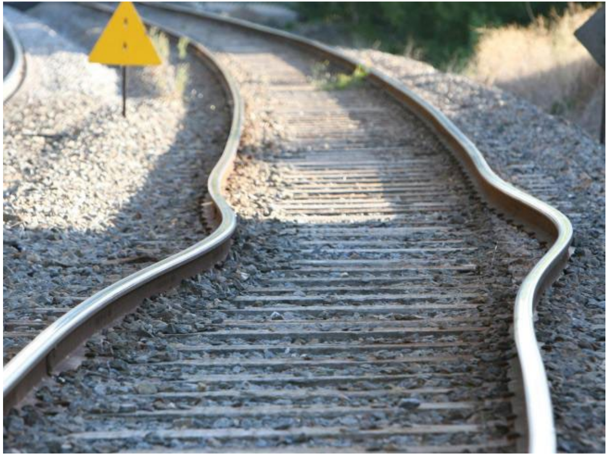
Prolonged exposure to extreme heat can produce kinking in the steel tracks of freight and urban transit rail systems.
