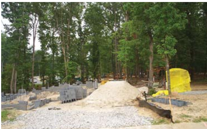
Figure 6. Improper disposal of construction materials and inadequate protection negatively impact trees at a construction site.
