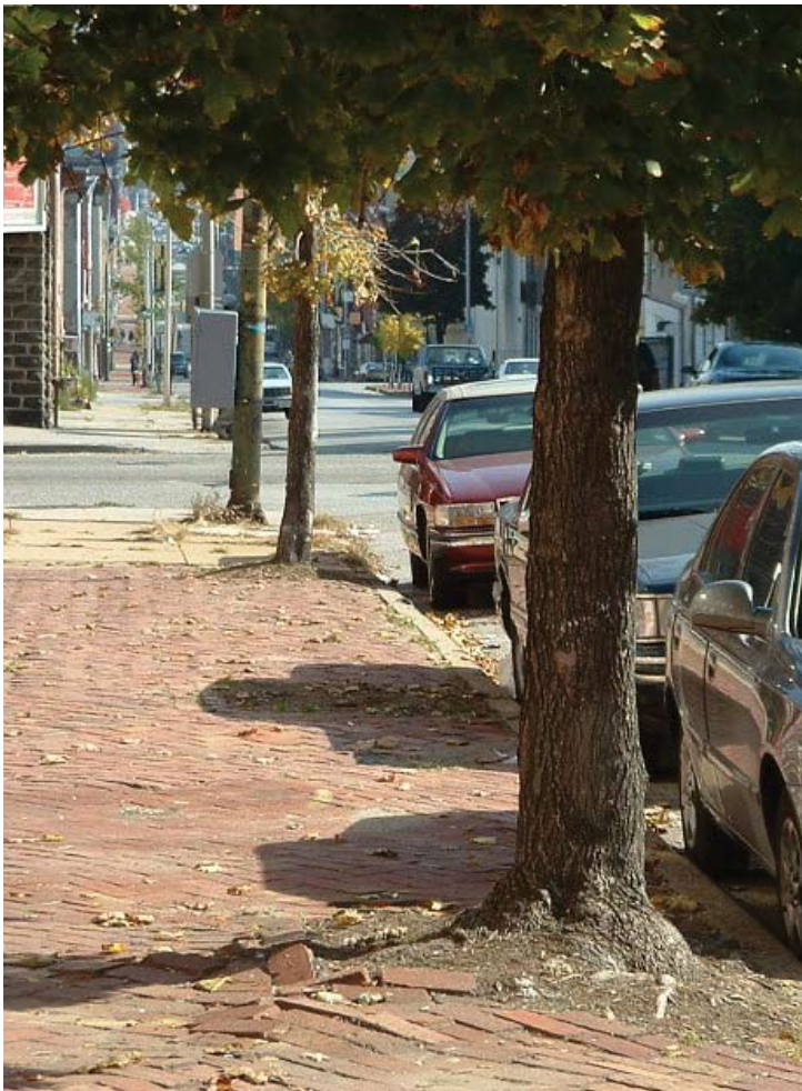
Figure 9. A common infrastructure conflict results in tree roots lifting or cracking pavement due to inadequate setbacks between trees and pavement.
