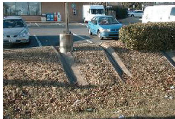
Directing runoff from impervious surfaces, such as parking lots, onto vegetated areas using curb cuts can achieve pollutant removal and reduce runoff quantity through infiltration
