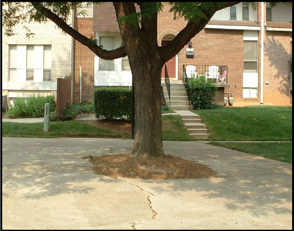
Figure 16. Tree roots cause adjacent pavement to crack
