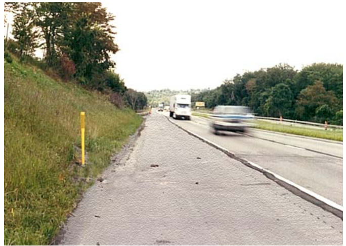
Porous paving and other cool paving products can be used for roadway shoulders to assist in runoff management while reducing the heat island effect.
