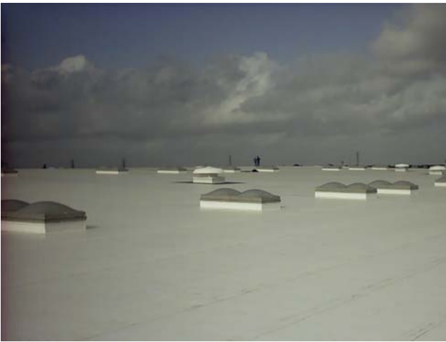
Reflective roofing installed on a University of Texas Health Science Center building in Houston.
