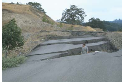
Figure 5.6: A road constructed on an unstable soil.
