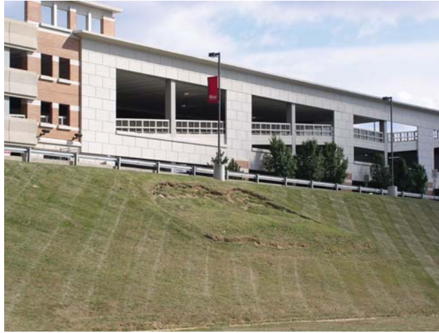
Figure 3.8: Soil slump on a steep slope below a mall.
