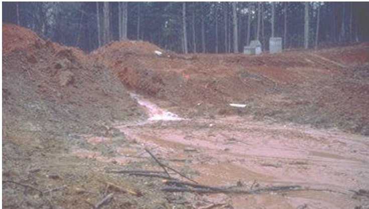
Construction activities can cause soil erosion.
