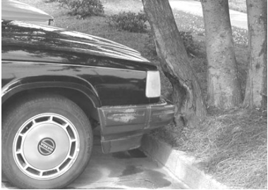
Inadequate tree protection from vehicles (photo by Mike Sherwood, Bartlett Tree Labs)
