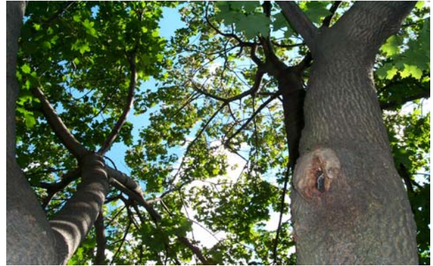
Fig.14. The thinning canopy on this Norway maple is the result of stem girdling roots (SGRs).
