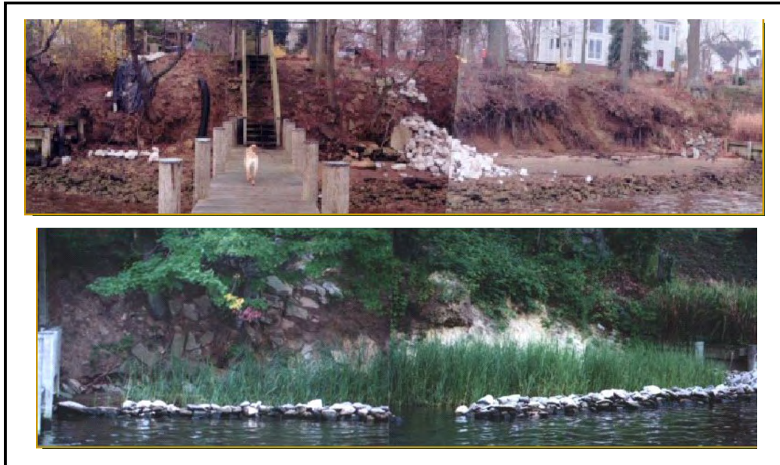
Figure 2. Before (top) and after (bottom) shots of a small shoreline restoration project. Here wetland plantings and rock sills were combined to prevent shoreline erosion. (Photos courtesy of South River Federation)
