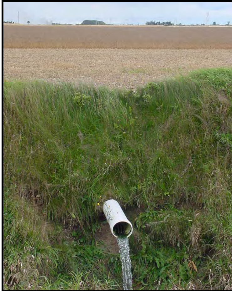
Figure 3. Drainage tiles are installed to convert wetlands to useable land for agriculture, a major cause of wetland loss (Source: Michigan State University Department of Geography)
