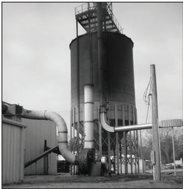
Figure 2. Dried wood shavings are kept in a storage silo that feeds the boiler. PHOTO COURTESY OF LAUREL LUMBER.
